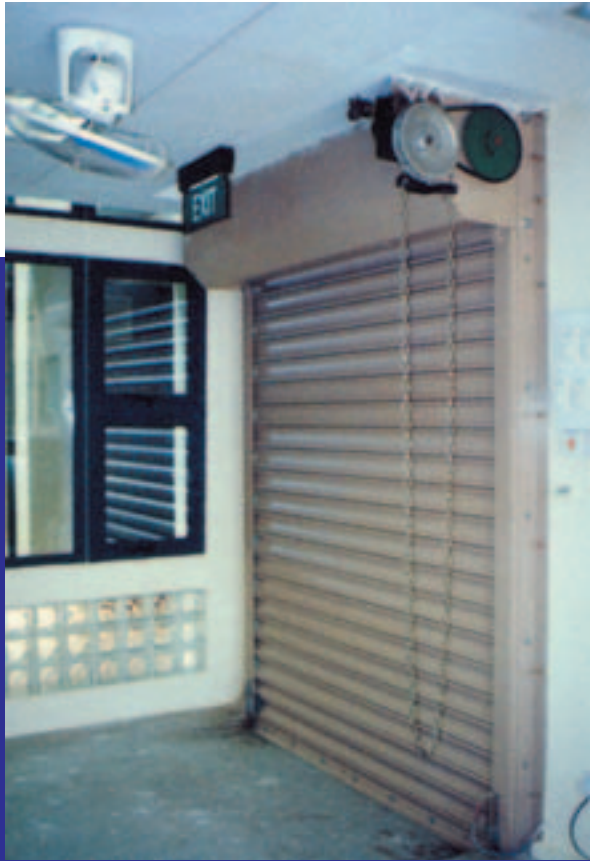
Fire Shutter with manual chain hoist
